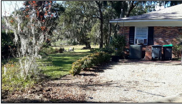
HVAC system not elevated
