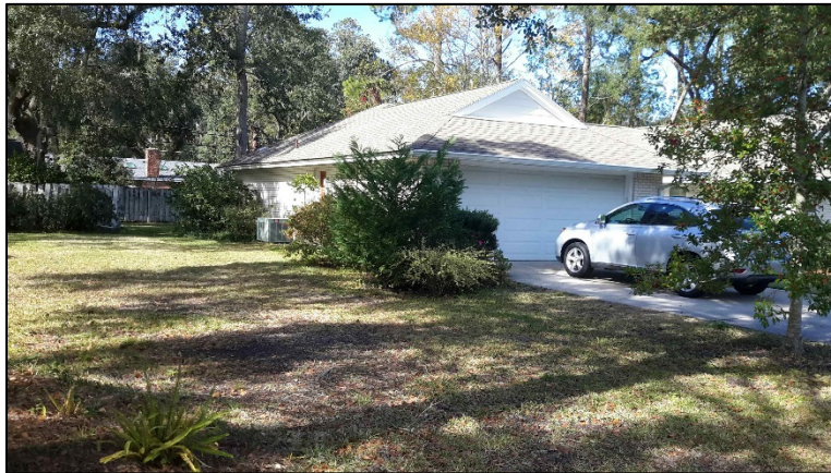
HVAC at grade
